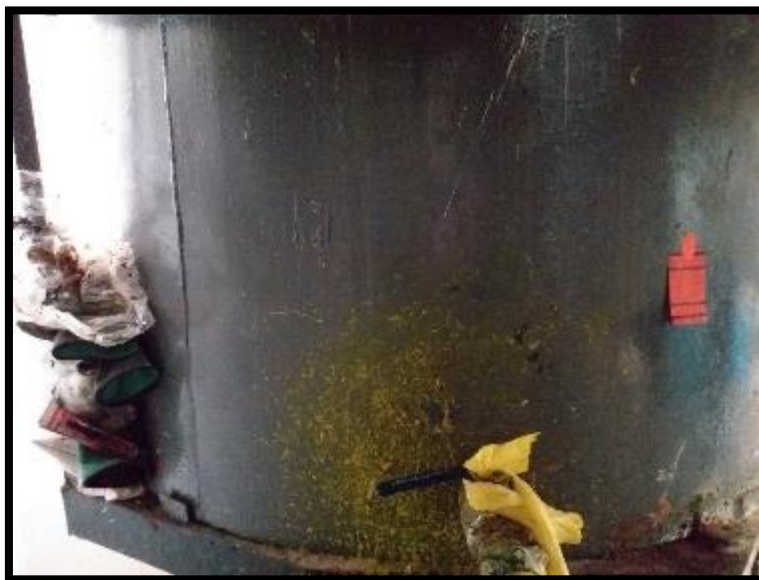
Figura 70 Tanque reactor No.2
